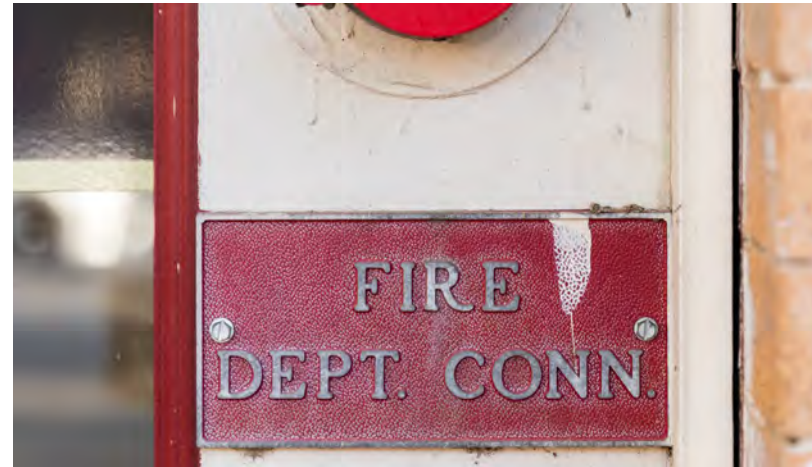
Fire Department connection on Main Street in Downtown Vacaville (Source: ESA)
