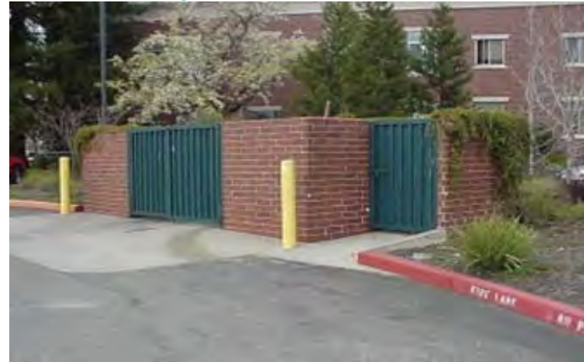
Appropriately screened service area with masonry and steel enclosure that matches the adjacent building (Source: Jacobs)
