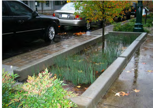
Figure 55 Median stormwater bio-retention area
