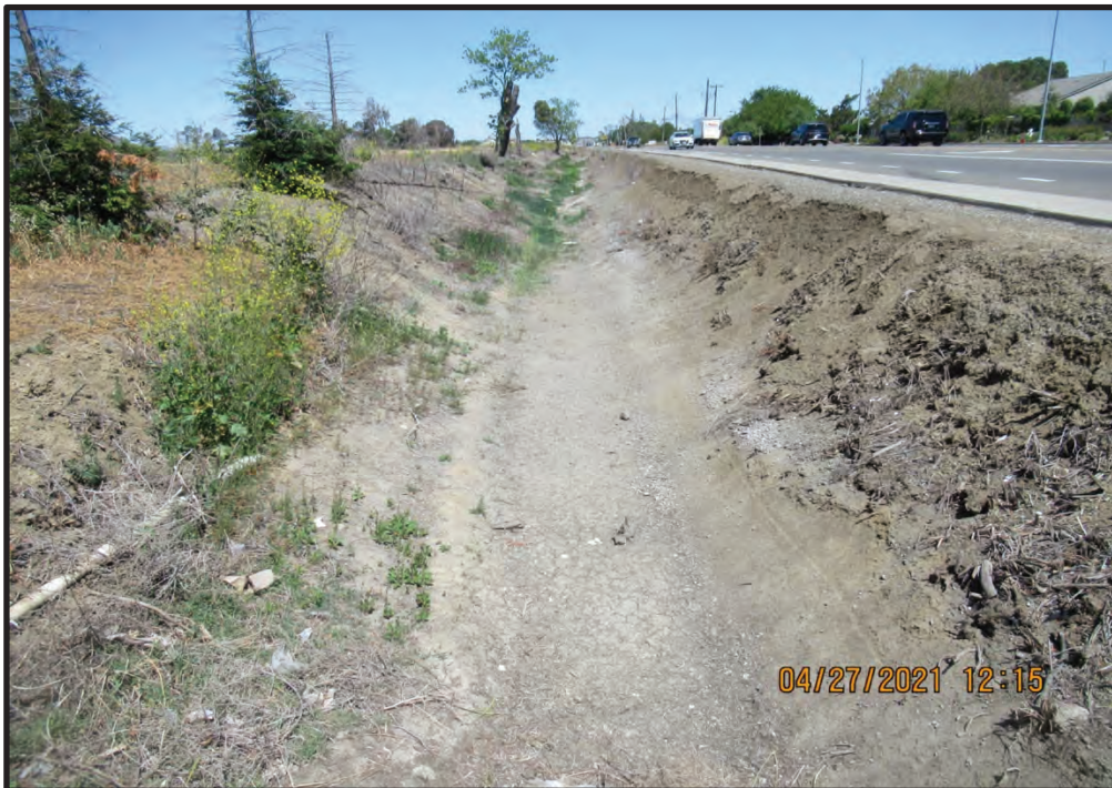
Constructed Ditch D-7, looking north along Leisure Town Road from adjacent to the City's sewer station; 04/27/21.
