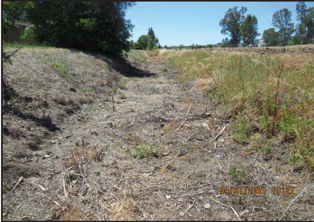
Constructed Ditch D-9, looking southwest; 04/27/21. This ditch carries storm water from the adjacent neighborhood to Pond P-2. Water from this ditch passes through the network of ponds and ditches and discharges to Old Ulatis Creek.
