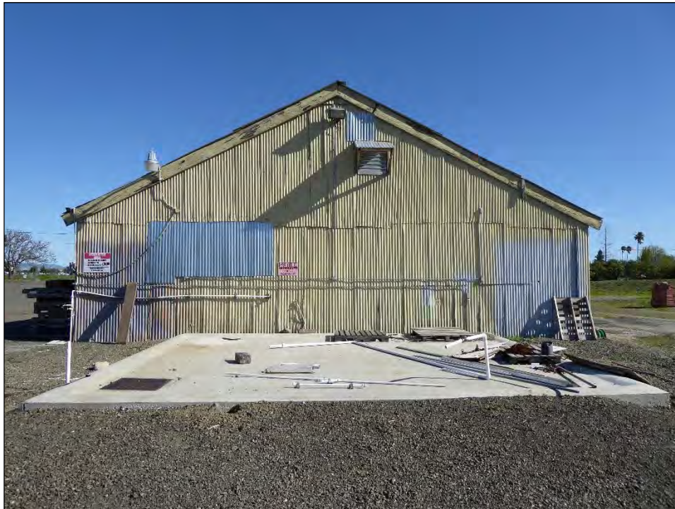
Photograph 16: South gable end of the warehouse, showing the concrete pad, camera facing north, April 12, 2019.
