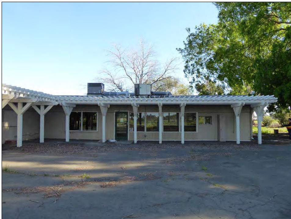
Photograph 3: View of fenestration on the south-facing section of the primary façade of the clubhouse, camera facing north, April 12, 2019.
