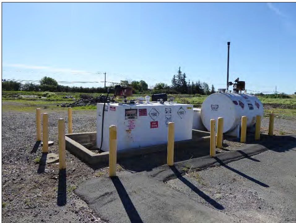
Photograph 19: Fueling station located south of the warehouse, camera facing south, April 12, 2019.
