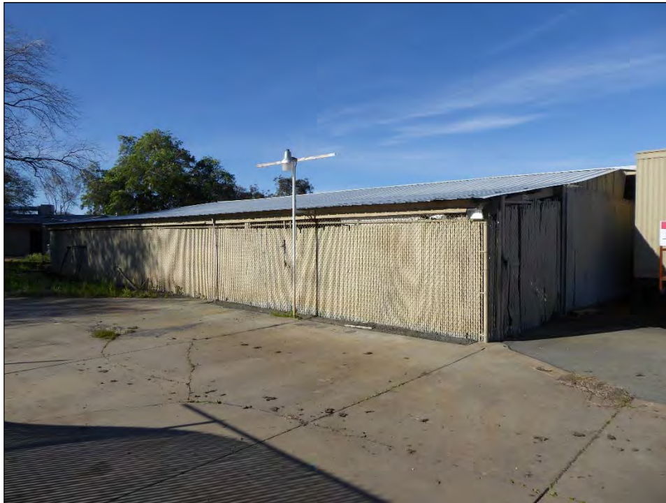
Photograph 10: View of the east side of the golf cart storage structure, enclosed by chainlink fencing, camera facing southwest, April 12, 2019.
