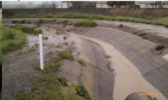
SID irrigation canal conveying overtopping storm water
