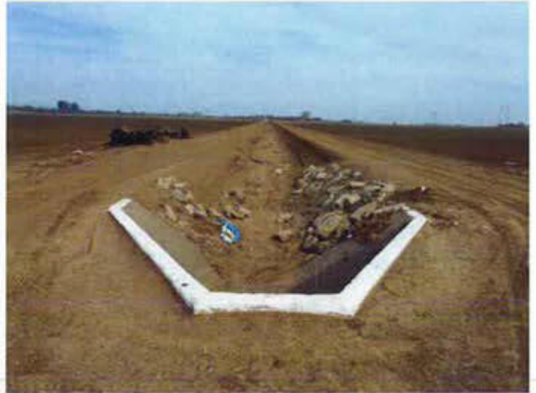
Photo 6. North-facing view of a water canal located on the central portion of the property.
